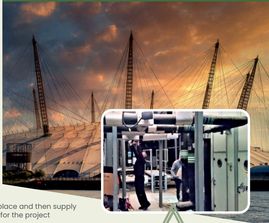
BVS engineers on-site carrying out a refurbishment of two large AHUs at The O2 London
