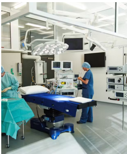
The AHU Supplied The Operation Theatres
