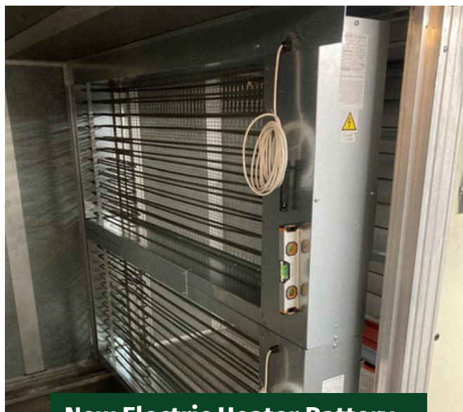
New Electric Heater Battery
